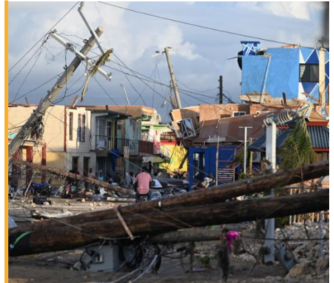
Hurricane Melissa heavily damaged infrastructure in Black River, St. Elizabeth Parish, Jamaica. Photo/Ricardo Makyn, AFP Images.
